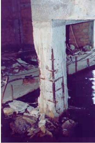
Corroded reinforcement behind spalling concrete
