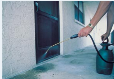
After the repaired area has dried sufficiently, the entire balcony surface is sprayed with Degussa Protectosil® CIT to protect it.
