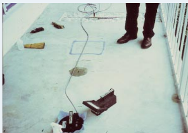
Moisture and chlorides caused corrosion on this balcony. Using linear polarization the corrosion rate is assessed.
