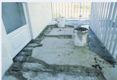
This damaged area is repaired and resurfaced.
